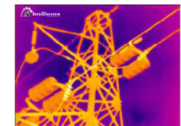
High voltage wire porcelain set overheating
