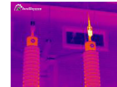
Sleeve connection overheating
